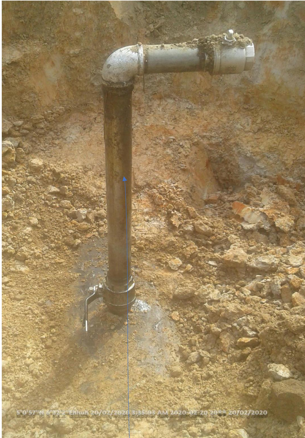
PIC: SHOWING POINT AFTER EXPOSURE (2" BALL VALVE AND 2 CALVANIZED PIPE WITH ELBOW AT 12'O CLOCK POSITION ON THE PIPELINE)
